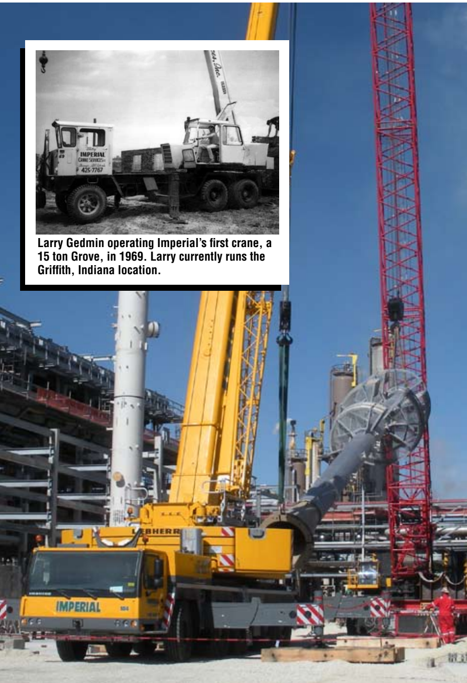
235 ton Liebherr works in tandem with 350 ton Sany crawler at CITGO refinery project.
